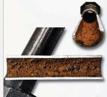
This actual cutaway of black iron compressed air piping shows typical contaminant build up and flow restriction after just a few years of operation.
